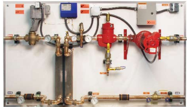
Typical Snow Melt Panel
